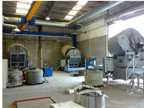
Three 1500kg.firing units in operation
